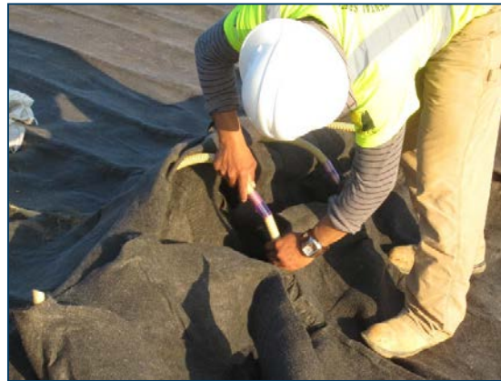
Figure 7: Mini-pipe junction with couplers
