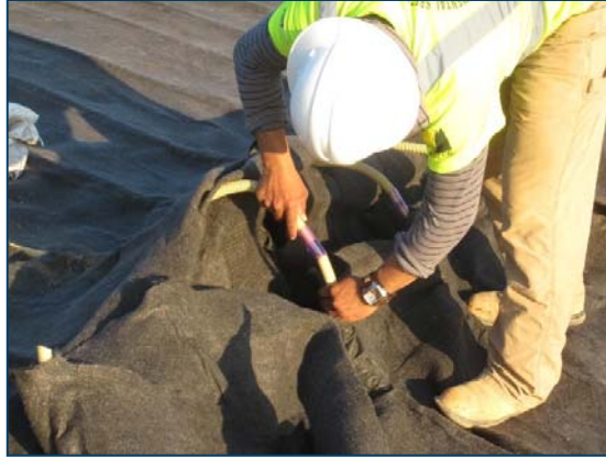
Figure 7: Mini-pipe junction with couplers
