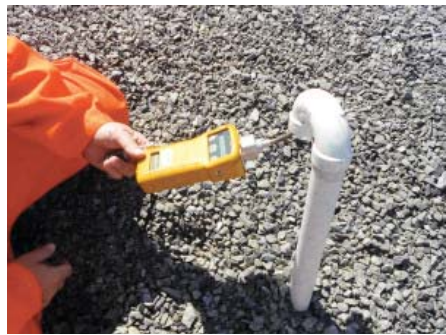
2A. Second surface impoundment at same site as shown previously having a geocomposite drain and proper venting with gas monitoring at one of the vents. Photos by GSI and Inova.
